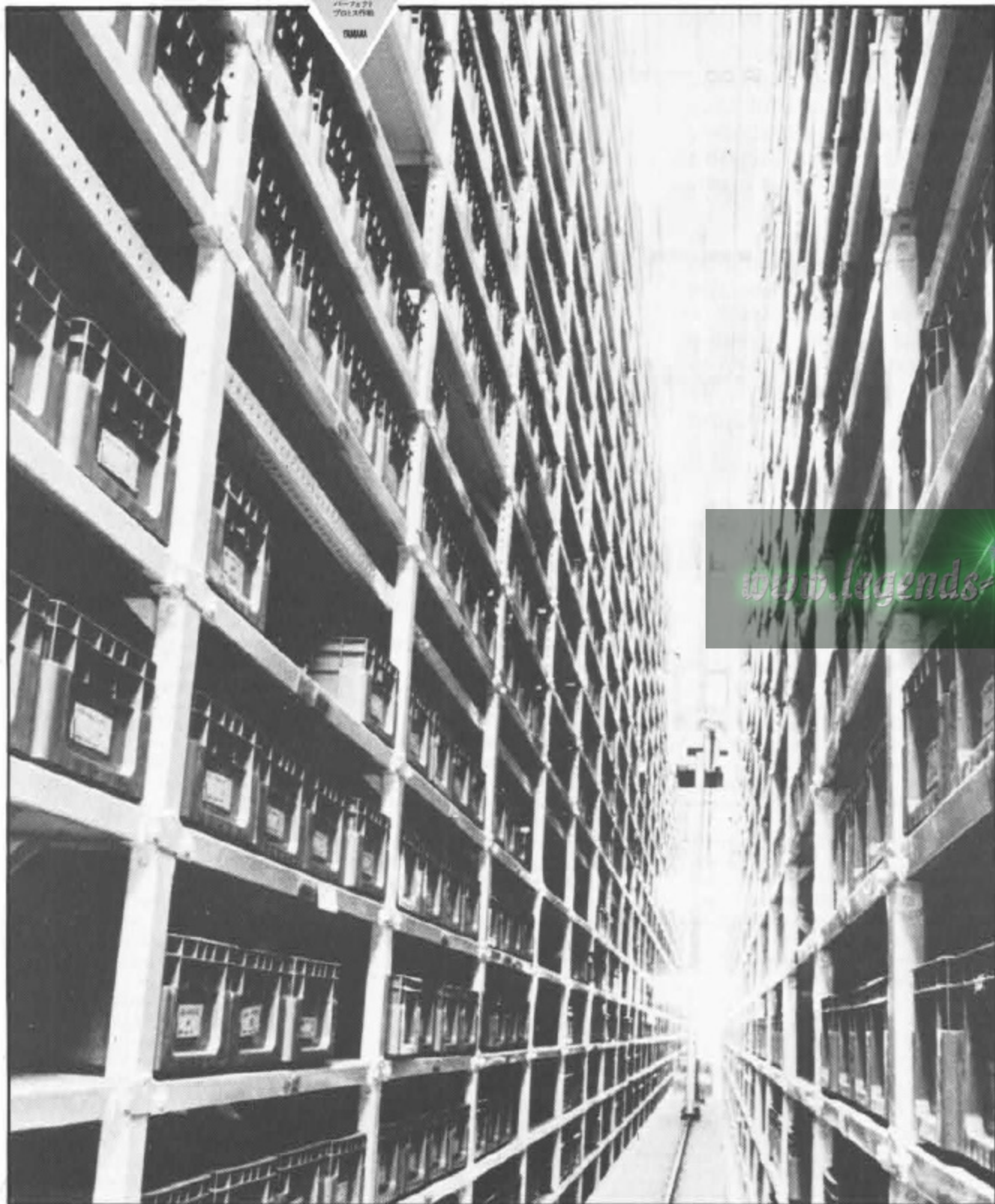
Lofty racks around which 8 stacker cranes are in constant action, are used for storing parts with high turnover rates.
