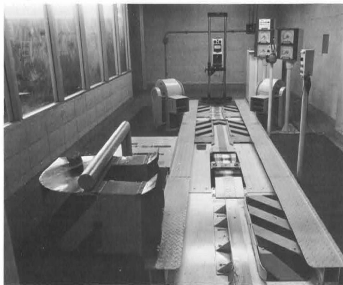
Diagnosis equipment is installed in a noise-proof room
