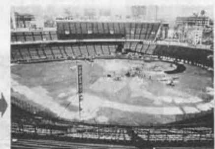
In addition to this, the area to be covered with dirt to become the track was laid over with yet another layer of plastic. No wonder that a total of about ten tons of plastic sheeting was used. Artificial dirt was hauled in with eleven-ton dump trucks and the bottom of the track was filled up first. Next, the quadruple jumps, the bank turns and the gap areas were fixed up with dirt. Anti-slipping material was fixed on the boards going up to the big jump and the descent from the jump was given dirt bumps.
