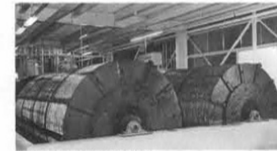
Water disposal equipment
